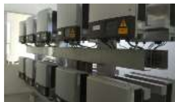
Gambar 3. 9 String Inverter SMA STP5000TL
