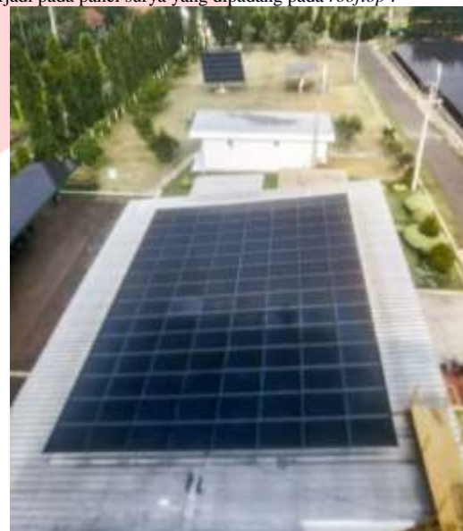
Gambar 4. 7 Rooftop Terkena Shading
