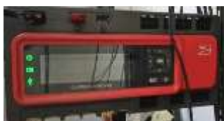
Gambar 3. 3 Data Logger (SMA CLUSTER CONTROLLER)
