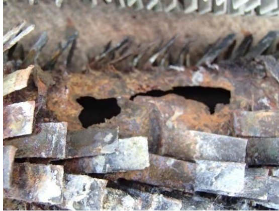
Gambar I.4 Lubang Penyebab Kebocoran Coil Heat Exchanger
