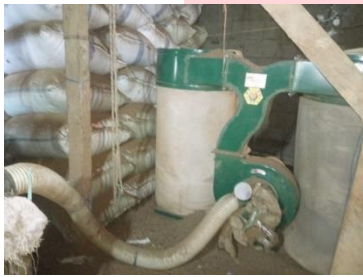
GAMBAR 3 Cyclone Dust Collector Existing
