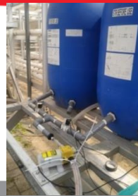
Figure 4.3. Pump and Water Tank Implementation
