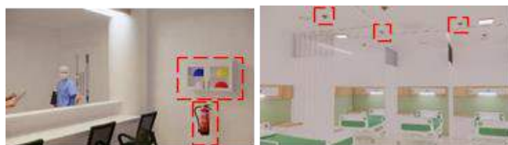
Gambar 18 APAR, APD disaster, springkler, dan smoke detector
