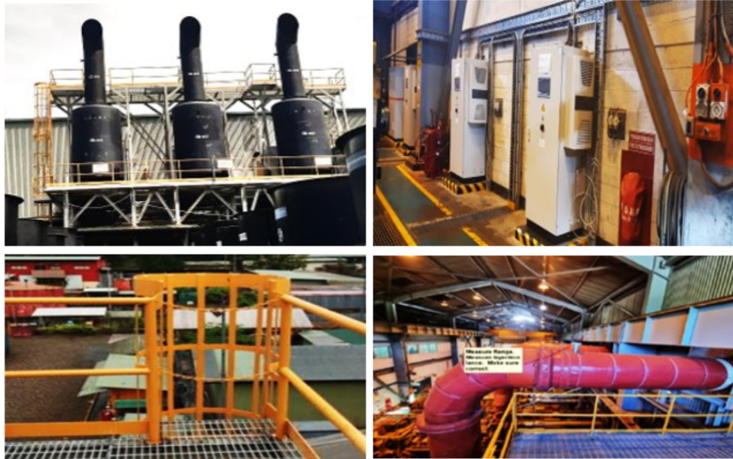
Gambar 1.6 Instalasi SCR Light Industrial Park (LIP)
